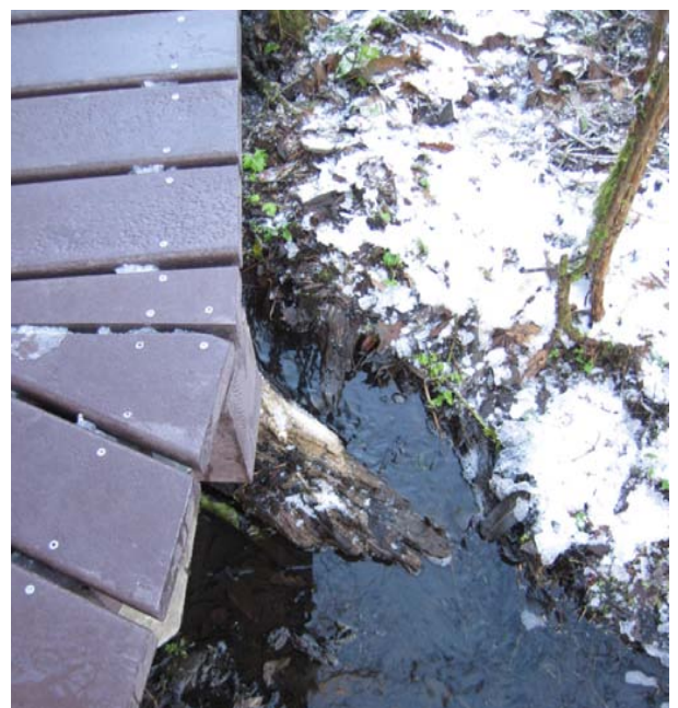
Water flow under the boardwalk is eroding the soil at this pin foundation .
