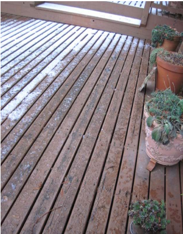
Here the deck remodel at my house blends smoothly with the previous deck structure.
