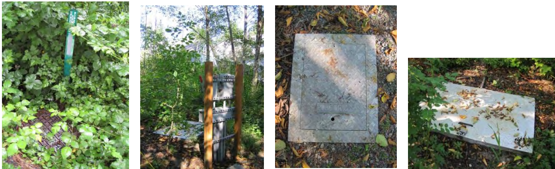
Photos 3.59-3.62: (L to R) Some of the site utilities that would need to be located and marked are near the gravel path in the northwest corner by the trout stream in sectors 161 and 183 (photos Hanson 2011).
