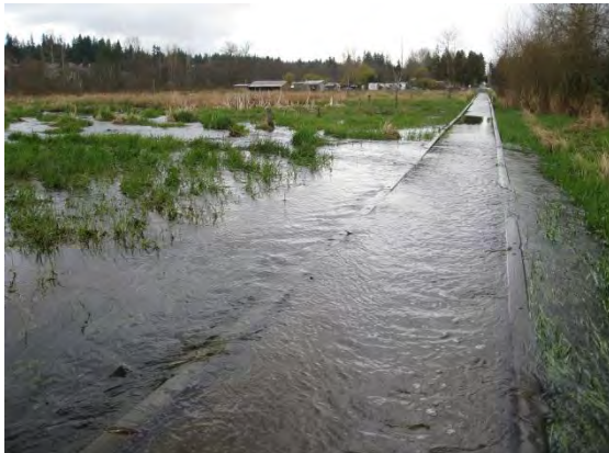
Photo 6.22: The boardwalk and stormwater interact In April 2011 (Hanson 2011)
