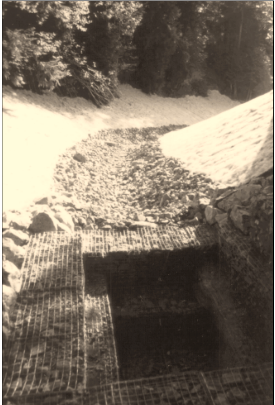
ENERGY DISSIPATOR AND STABILIZED CHANNEL IN HILTON LAKES DRAINAGE, PHOTO BY JOHN ENGEL
